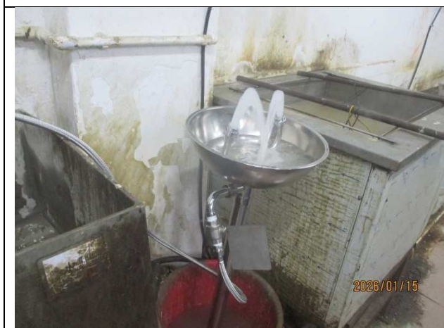
Eye wash station
